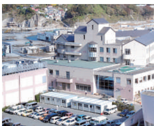
女川町立病院復旧工事 (電気設備) Repairs to the electrical facilities of Onagawa Hospital
