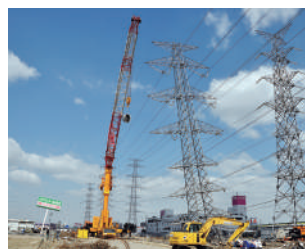
仙台港地区における被災送電鉄塔 撤去および復旧工事 Removal of and repairs to affected transmission line towers located in the Sendai Port area
