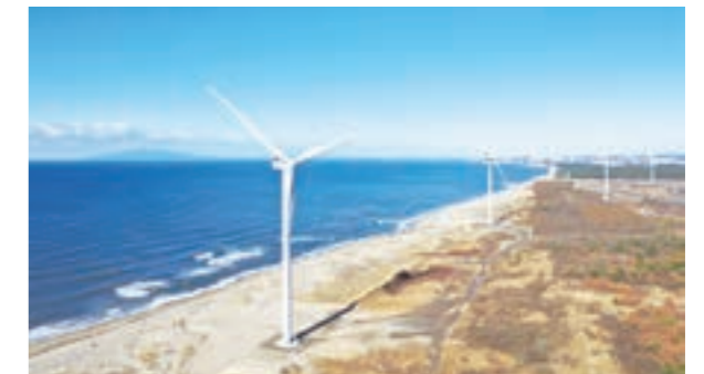
Akita Araya Wind Farm (Akita Prefecture)
