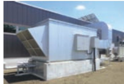
High-efficiency heat pump external air conditioner
