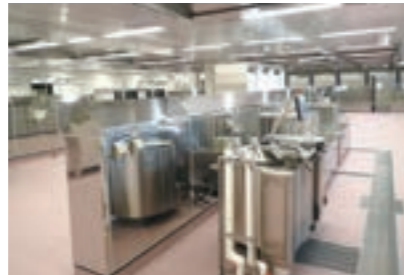
Kitchen equipped with a ceiling ventilation system (top of the photo)
